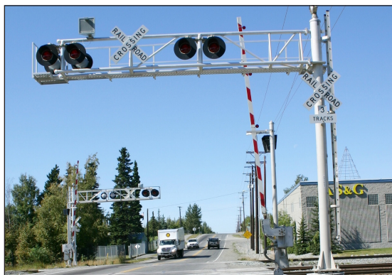
Automated wayside horns at Klatt Road crossing.
