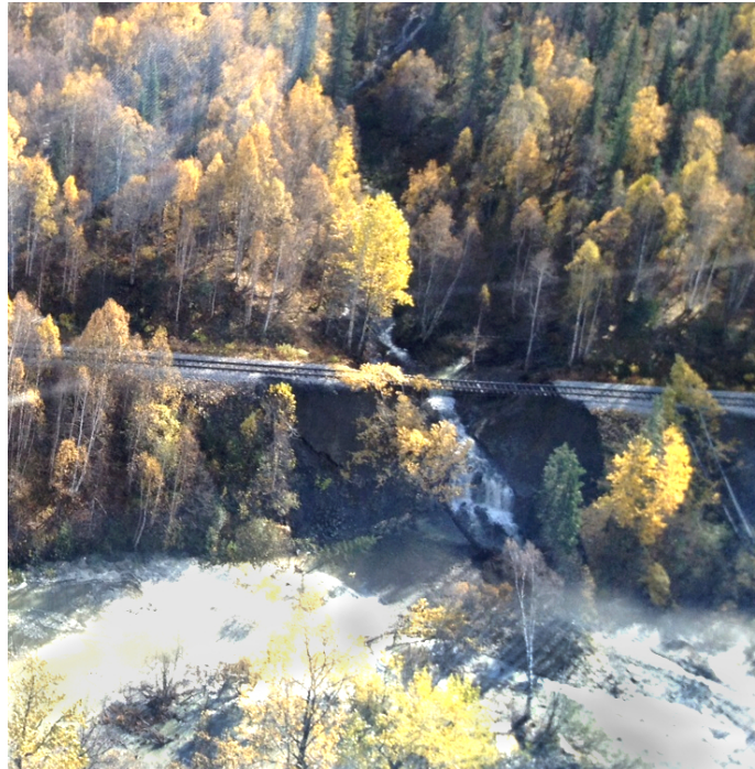
Major washout just south of Gold Creek.
